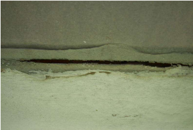
Open wall joint.
