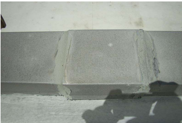
Open wall joints.
