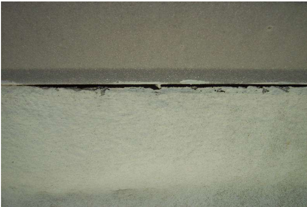
Open wall joint.
