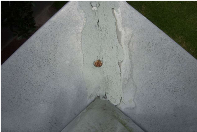
Open coping joint.
