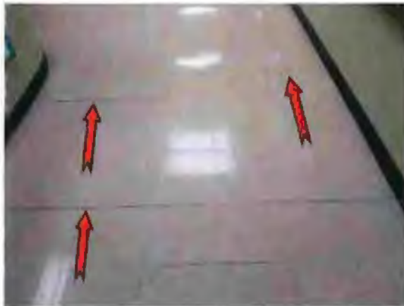
Photo #45 Separations in vinyl tile floor
