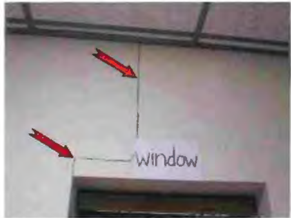
Photo #58 Crack in gypsum wallboard wall
