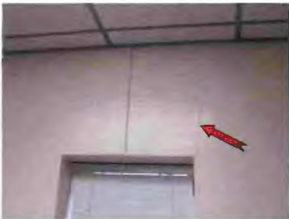
Photo #71 Crack in gypsum wallboard wall
