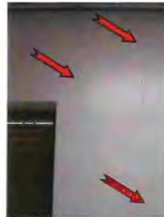
Photo #64 Cracks in gypsum wallboard wall
