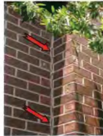
Photo #14 Separation at expansion joint
