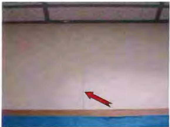
Photo #72 Crack in gypsum wallboard wall
