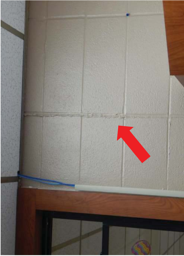
#50 Vertical crack in CMU wall
