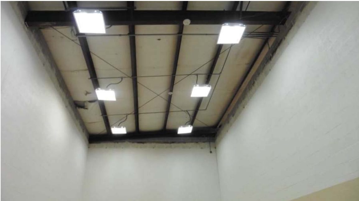
Examples of damaged “over-the-purlin” gym roof insulation
