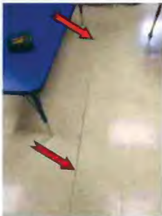
Photo #69 Separations in vinyl tile floor
