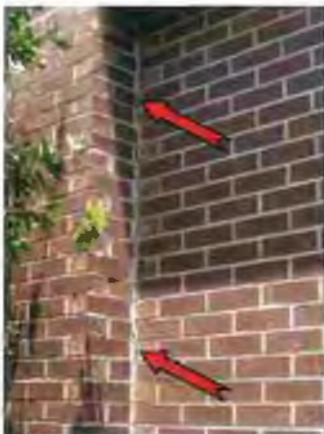
Photo #17 Separation at expansion joint
