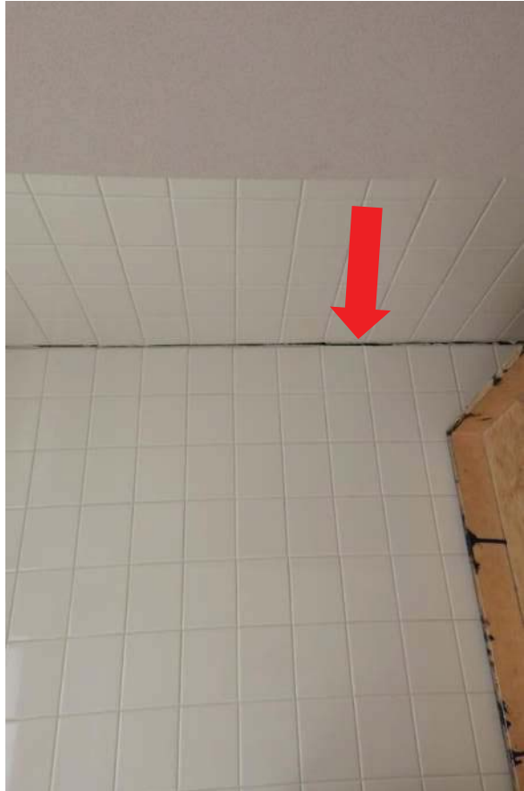
#37 Cracking and separation in tile
