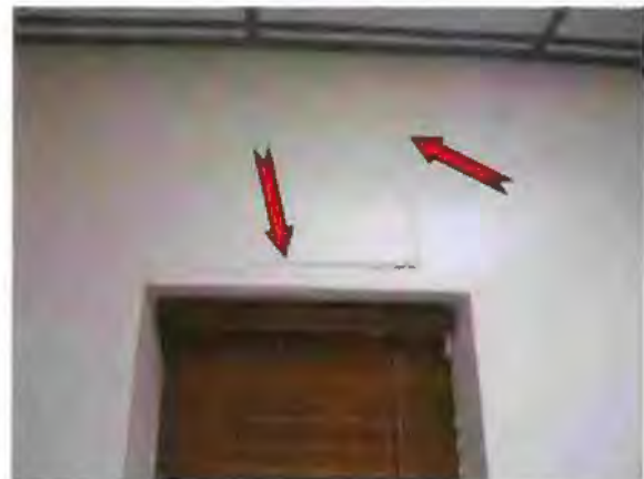
Photo #66 Crack in gypsum wallboard wall
