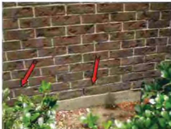
Photo #22 Masonry-mortar-joint crack
