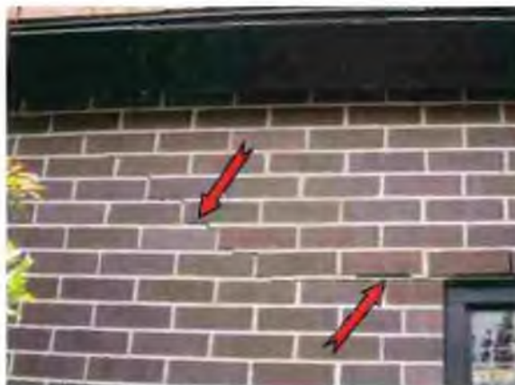
Photo #20 Masonry-mortar-joint crack
