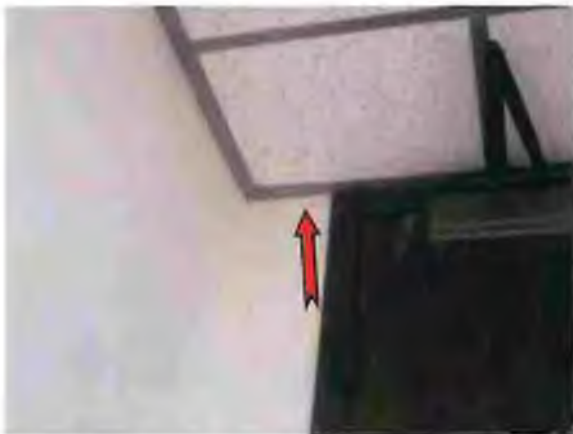
Photo #47 Crack in gypsum wallboard wall
