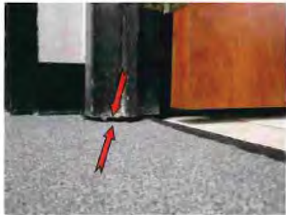
Photo #26 Separation between door frame and floor
