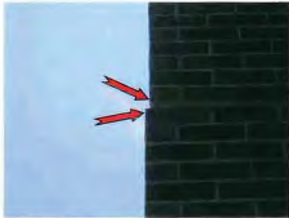
Photo #13 Lateral movement in brick veneer
