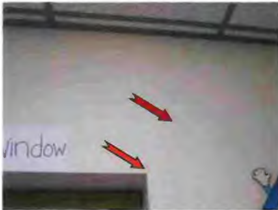
Photo #57 Crack in gypsum wallboard wall
