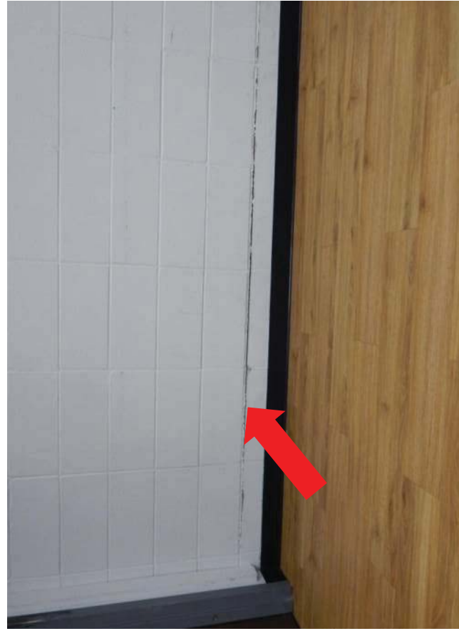
#46 Horizontal crack at base of CMU wall
