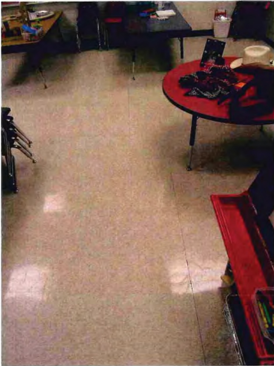
Photo 2. Separation of floor tiles in addition.
