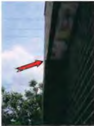
Photo #15 Lateral movement in brick veneer
