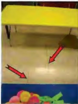
Photo #61 Separations in vinyl tile floor
