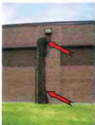
Photo #23 Staining on exterior brick veneer
