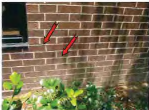
Photo #19 Masonry-mortar-joint crack
