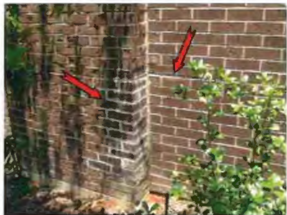
Photo #21 Masonry-mortar-joint crack
