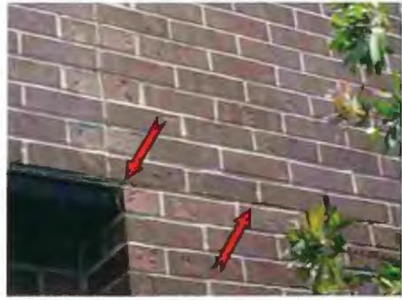
Photo #16 Separation at expansion joint
