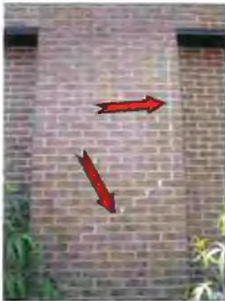
Photo #9 Masonry-mortar-joint crack
