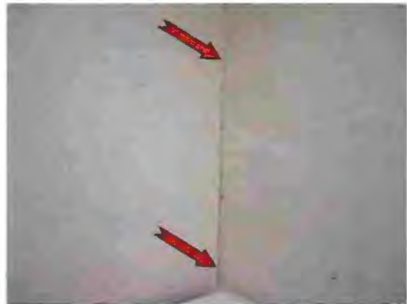
Photo #56 Crack in gypsum wallboard wall
