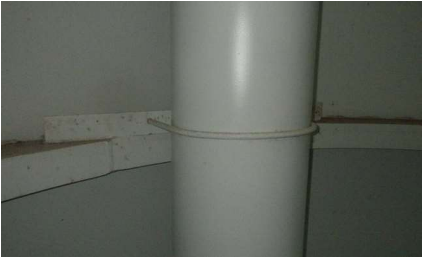
67. Inlet/outlet pipe U-bolted to bracket attached to the support column stiffener.
