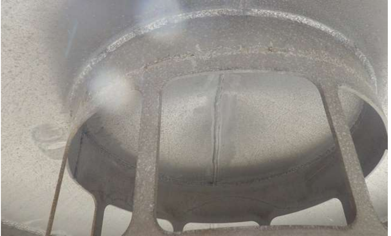
46. Roof vent missing screening.
