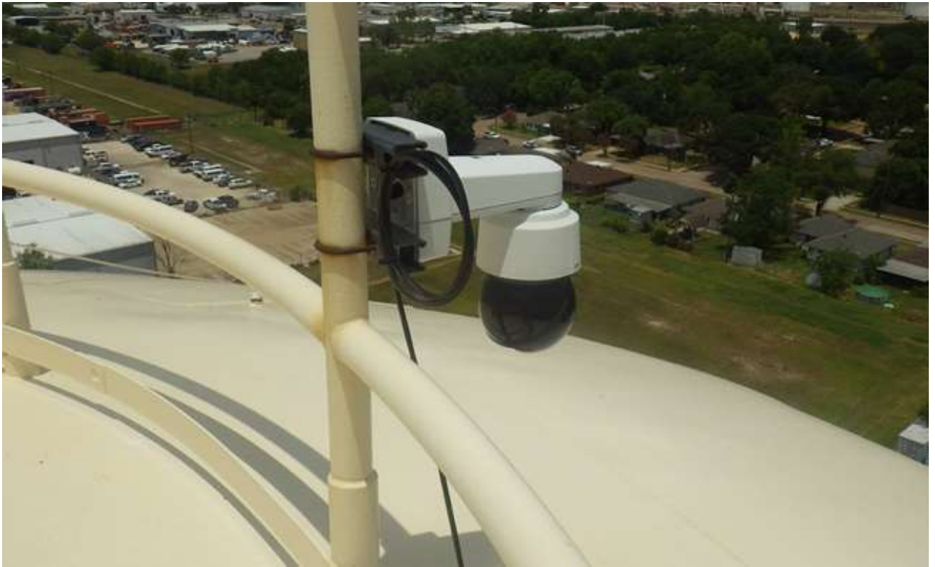
35. Surveillance camera attached to the roof safety railing.
