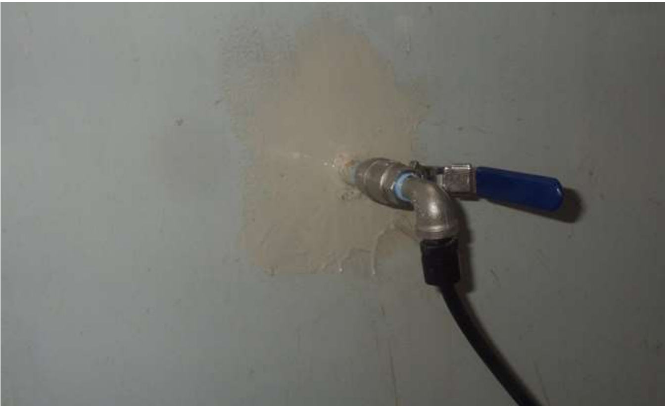
78. Touched-up area around pipe equipped with a valve penetrating the access tube.
