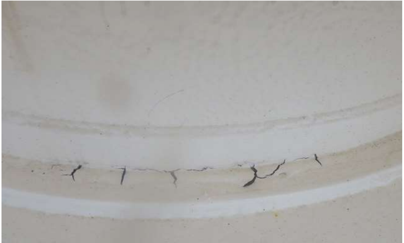
38. Coating failure around the access tube roof manhole curb.
