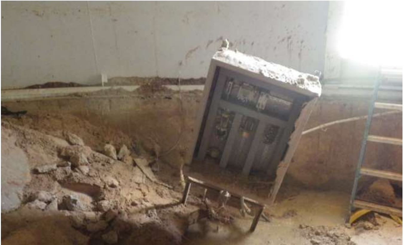
52. Uncovered electrical cabinet exposing wiring above severely damaged base cone floor.
