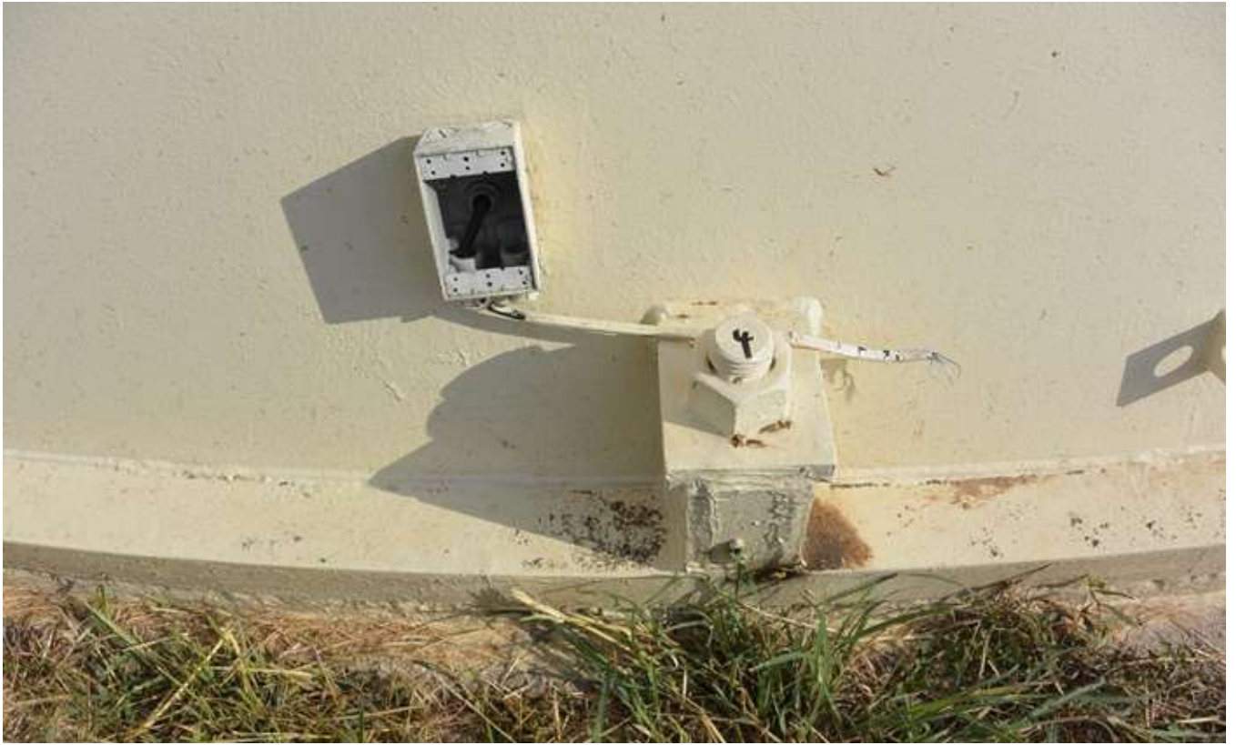
11. Uncovered conduit junction box and broken conduit exposing wiring.
