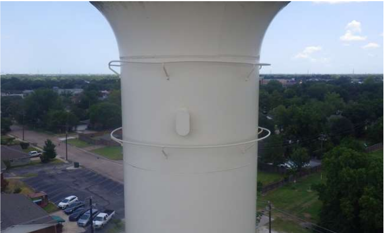
18. Painter's manhole and painter's rings near the top of the support column. Note bent painter's ring.
