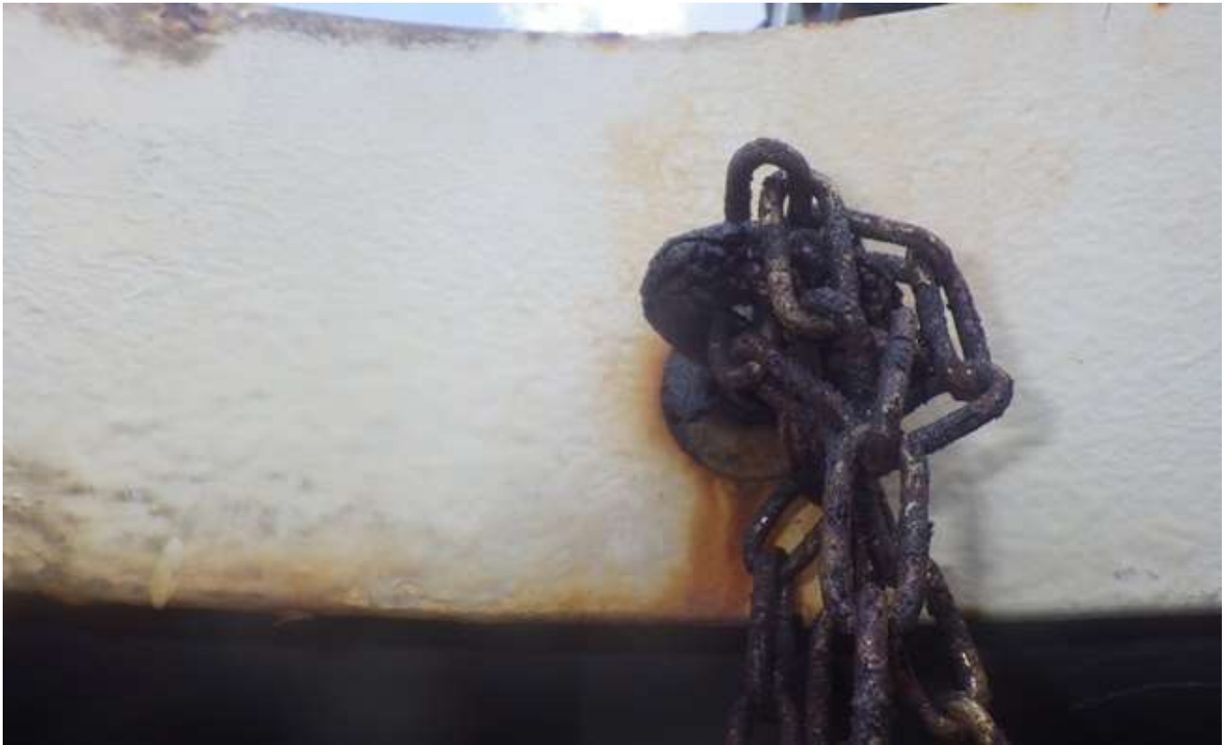
43. Corrosion and metal loss on chain penetrating the container roof manhole curb.
