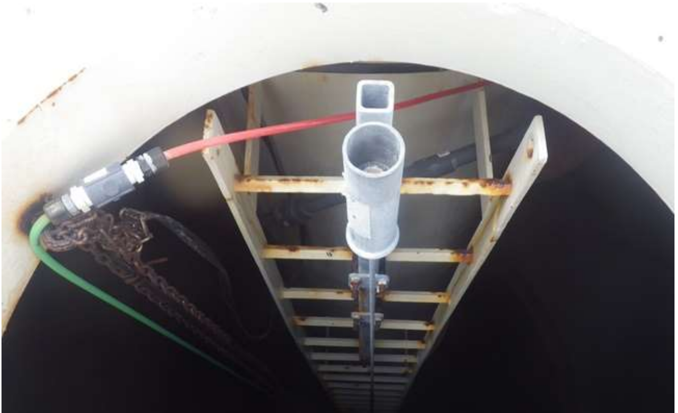
97. Interior wet container ladder rungs, safe-climbing device, and chains. Note corrosion on areas of the ladder rungs and on the chains.
