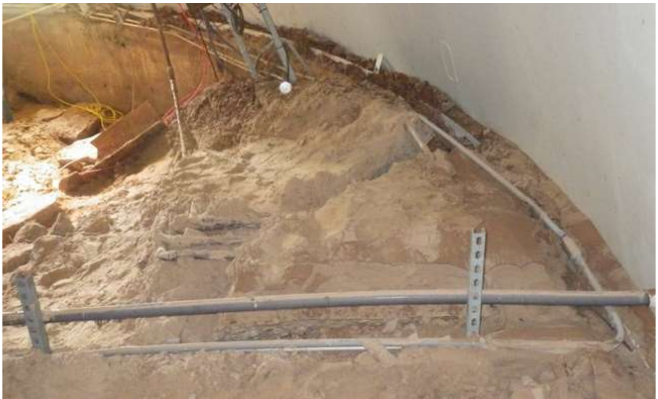
54. Conduits above severely damaged base cone floor.
