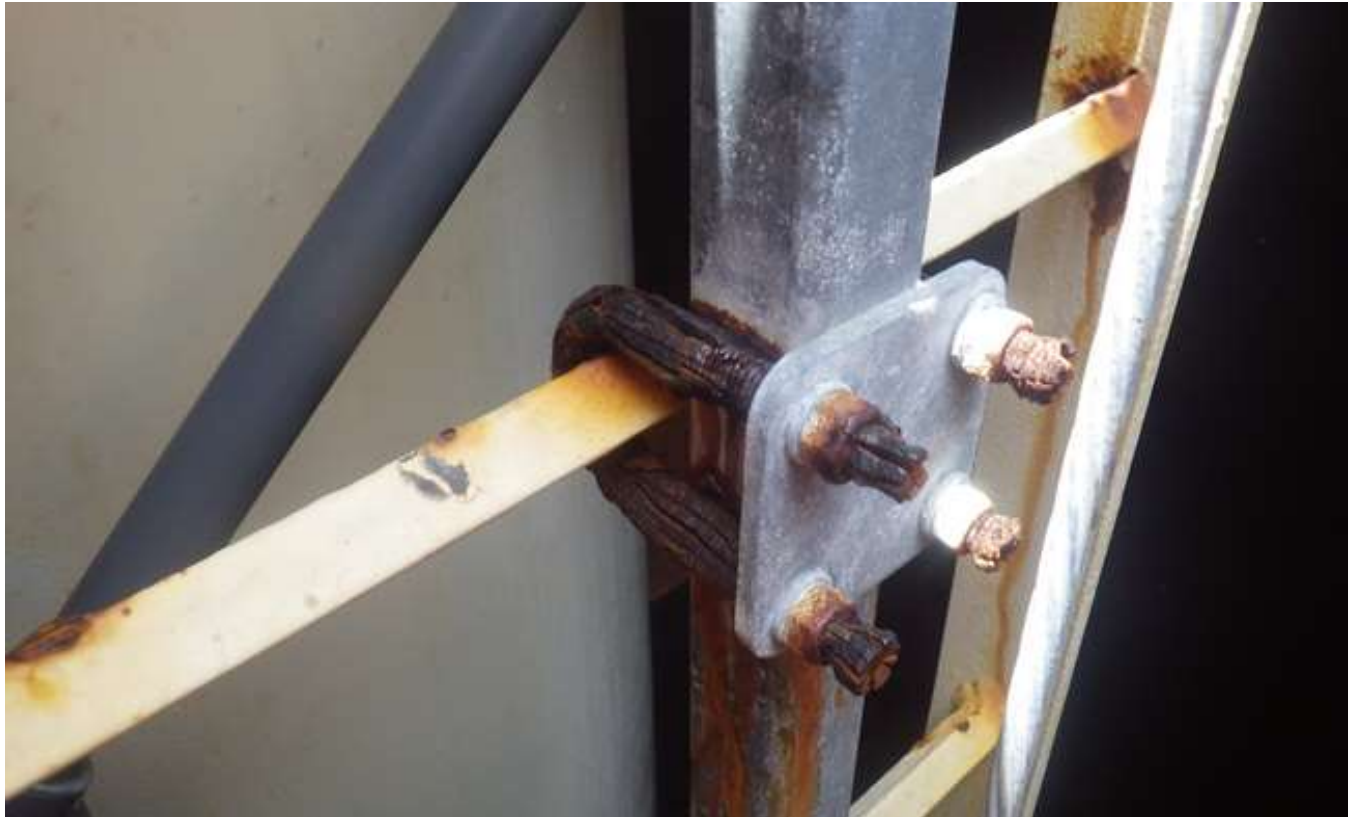
98. Corrosion and metal loss on the interior wet container ladder safe-climbing device bracket.
