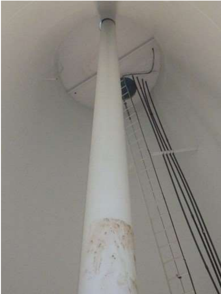
61. Inlet/outlet pipe extending up the base cone and through the condensate platform.
