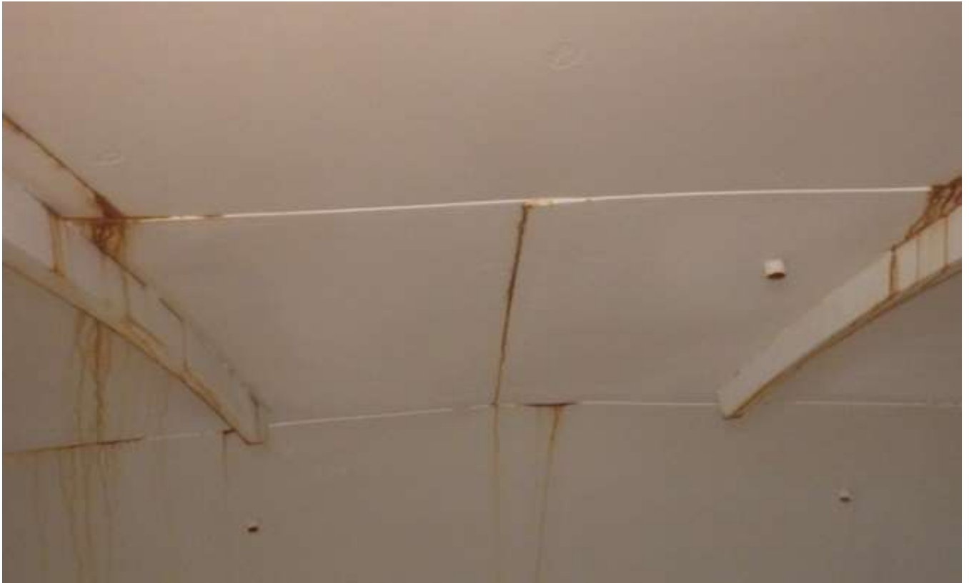
84. Corrosion and rust staining on areas of the roof interior and stiffeners.
