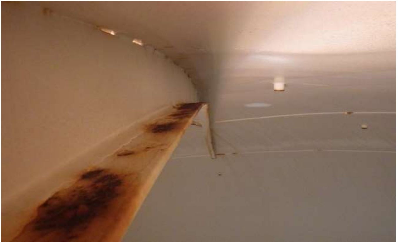
85. Corrosion on interior roof stiffener.
