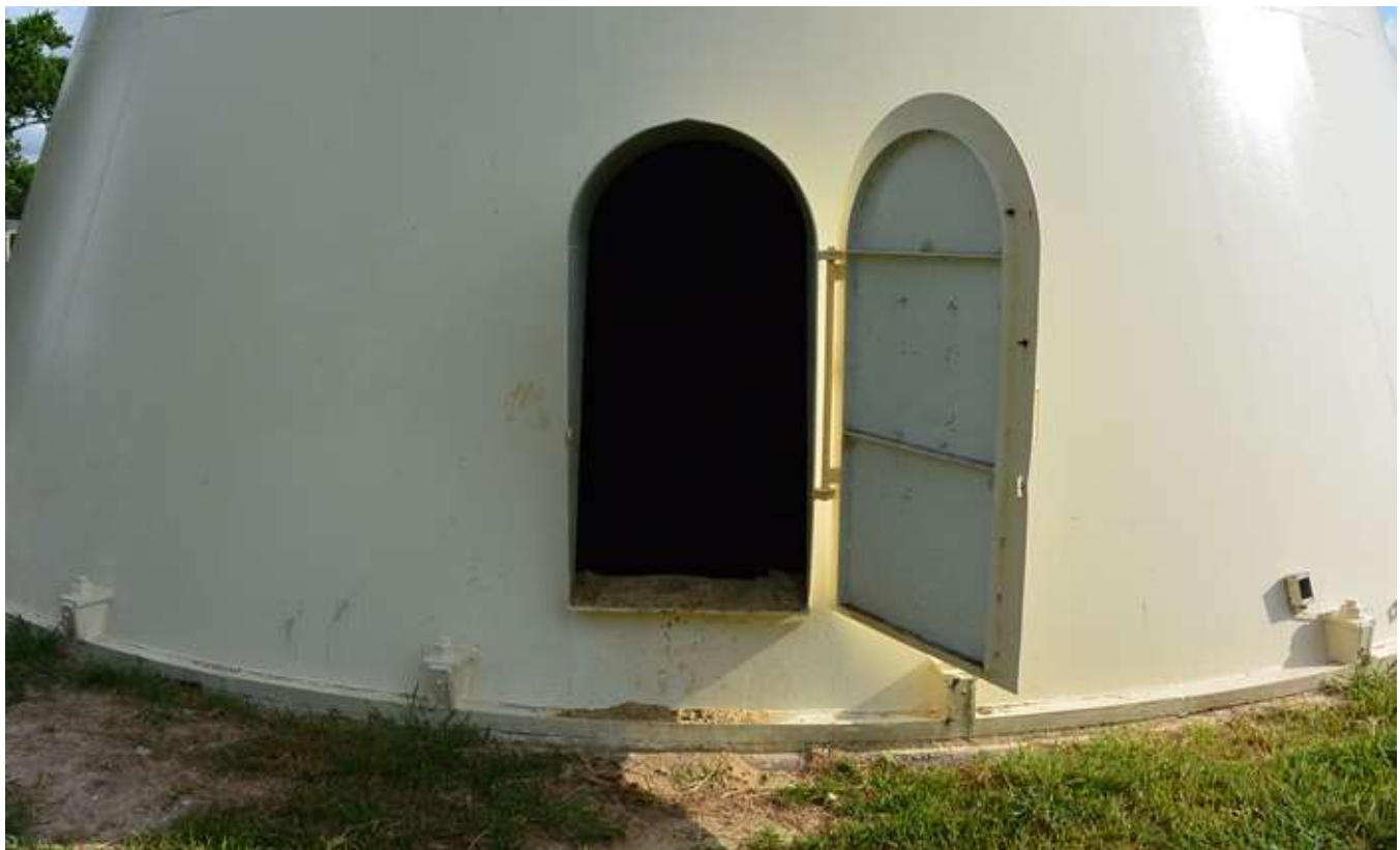
14. Base cone access door.
