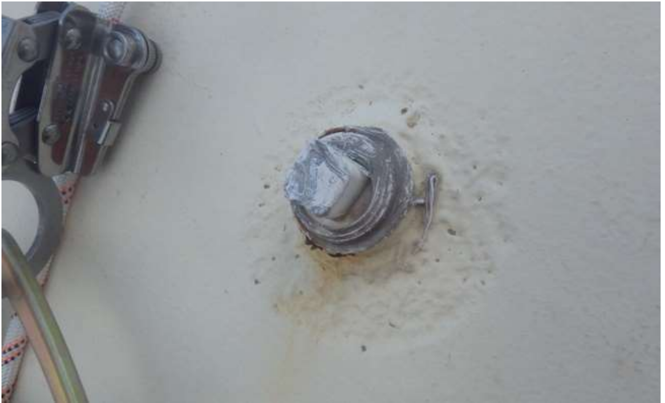
33. Pitting which had occurred prior to the last repainting around threaded and plugged coupling in the roof.
