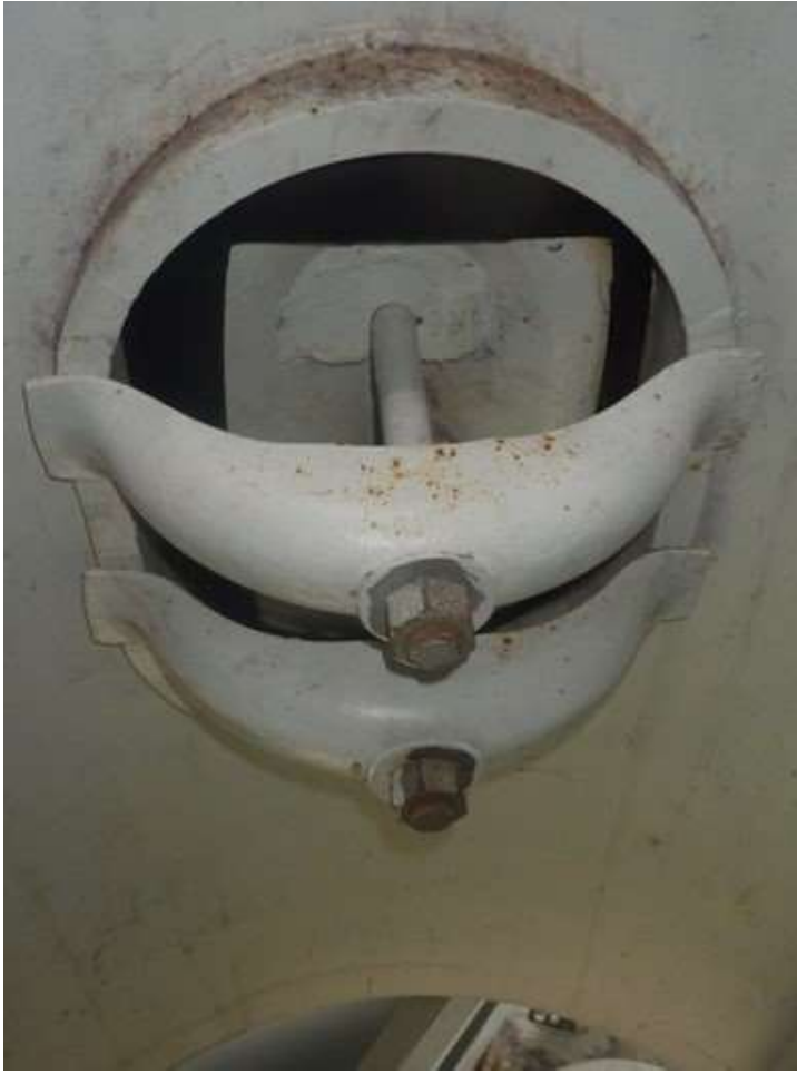
77. Access tube ventilation manhole.
