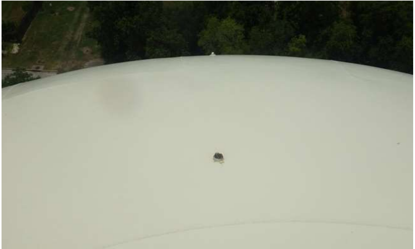
30. Roof exterior. Note corrosion on open coupling in the roof.
