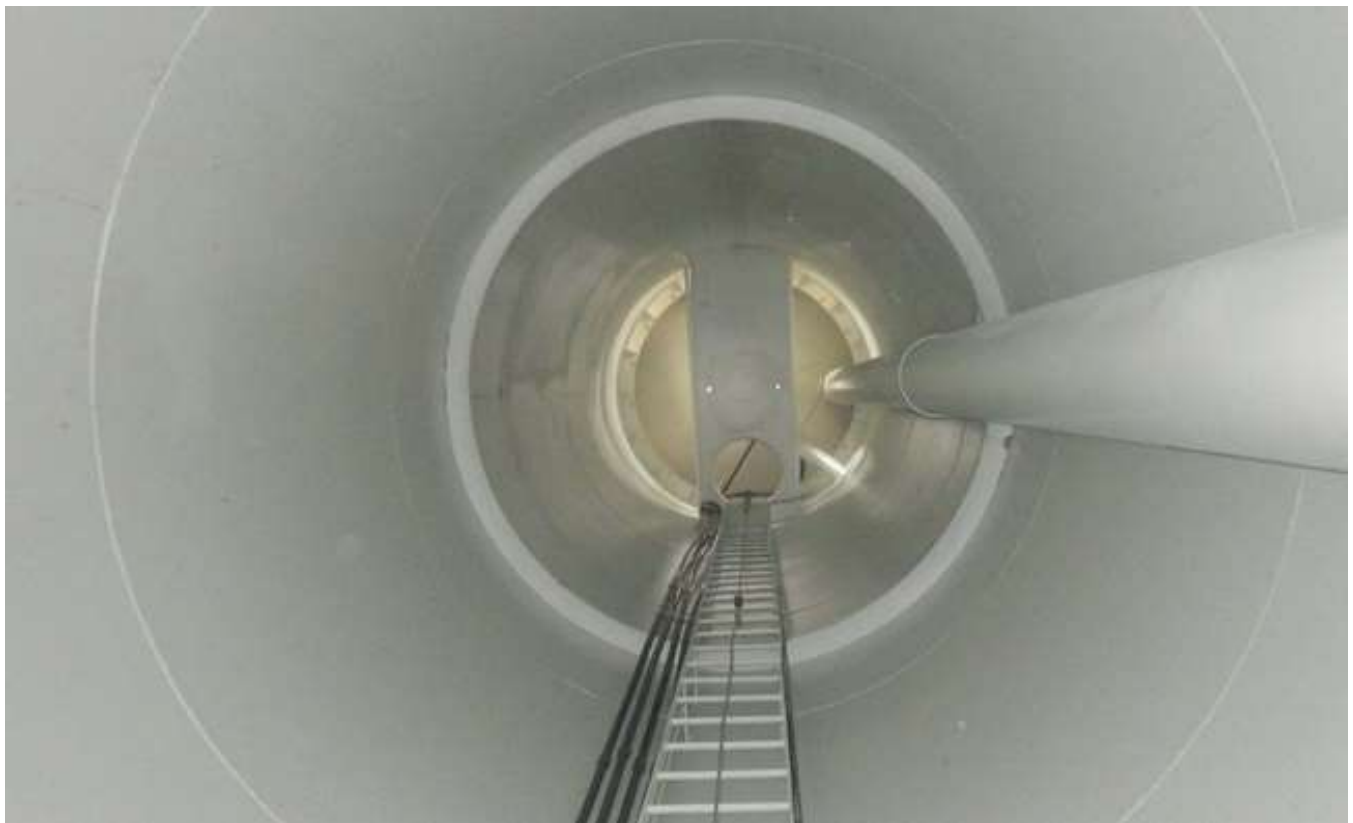
70. Support column ladder, safe-climbing device, cables, inlet/outlet pipe, and top platform.
