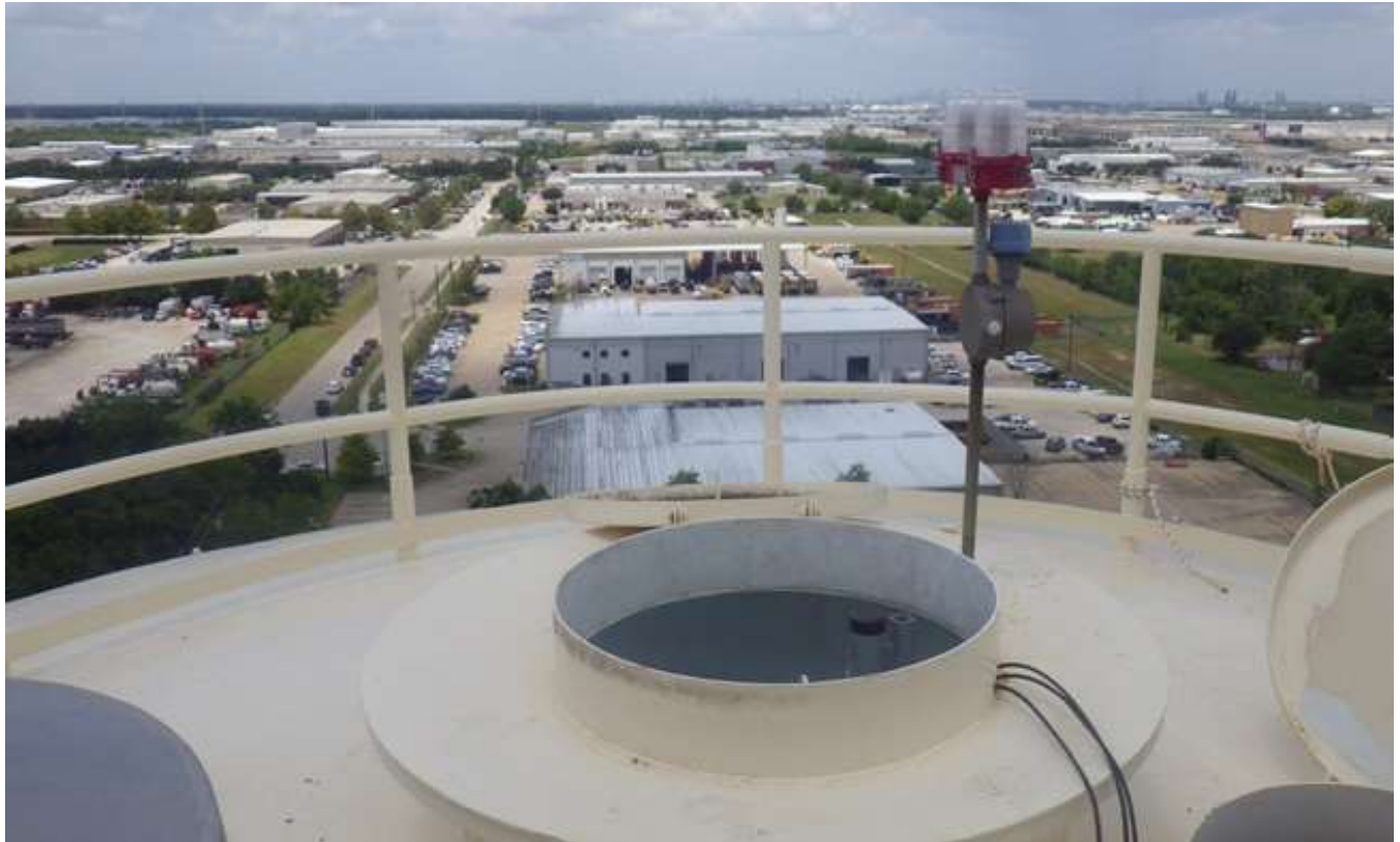
36. Roof safety railing, access tube roof manhole, and roof obstruction lights. Note cables extending through the manhole curb.
