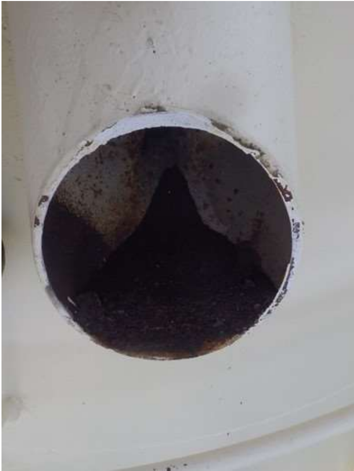
21. Corrosion on the interior of the overflow pipe discharge.
