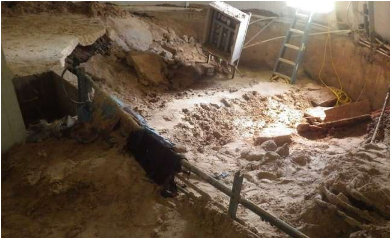
47. Conduits and cabinets exposing wiring at the severely damaged base cone floor.
