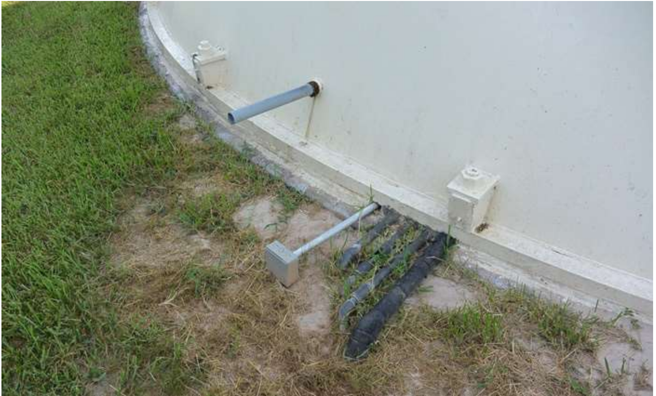
7. Conduits and piping extending from below grade and penetrating the foundation and pipe projecting from near the bottom of the base cone.
