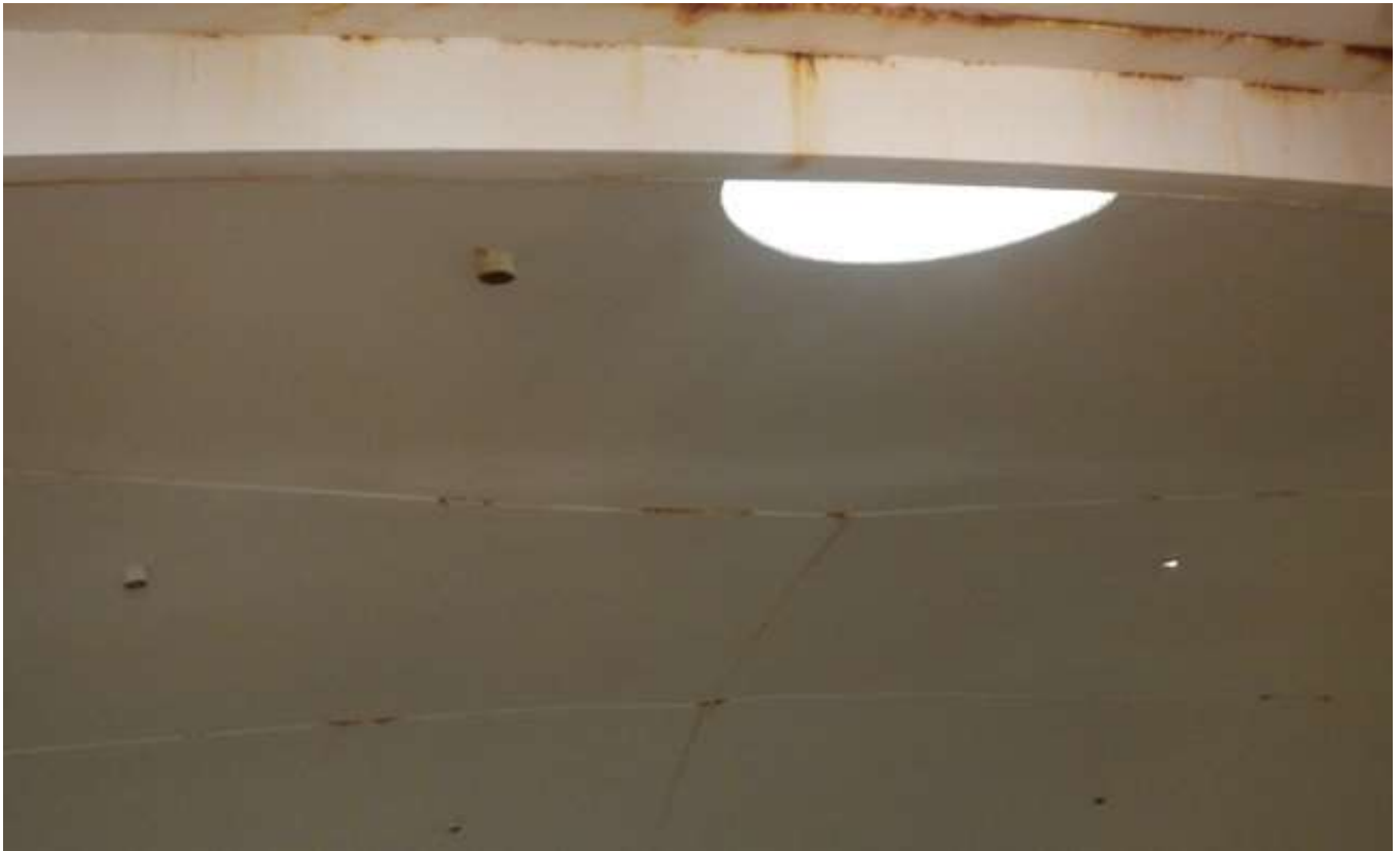
87. Corrosion and rust staining on areas of the roof interior and stiffener.
