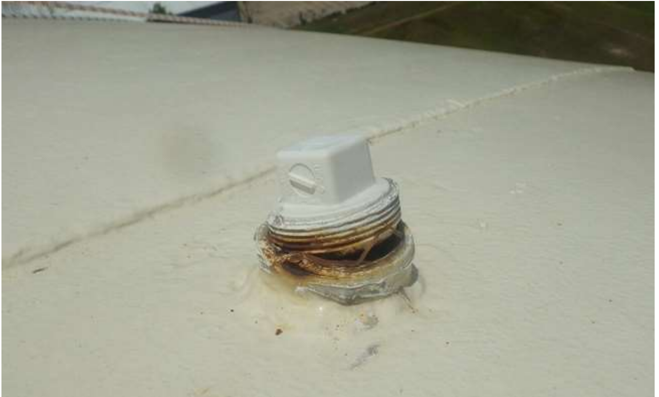
32. Broken plug of threaded and plugged coupling in the roof.
