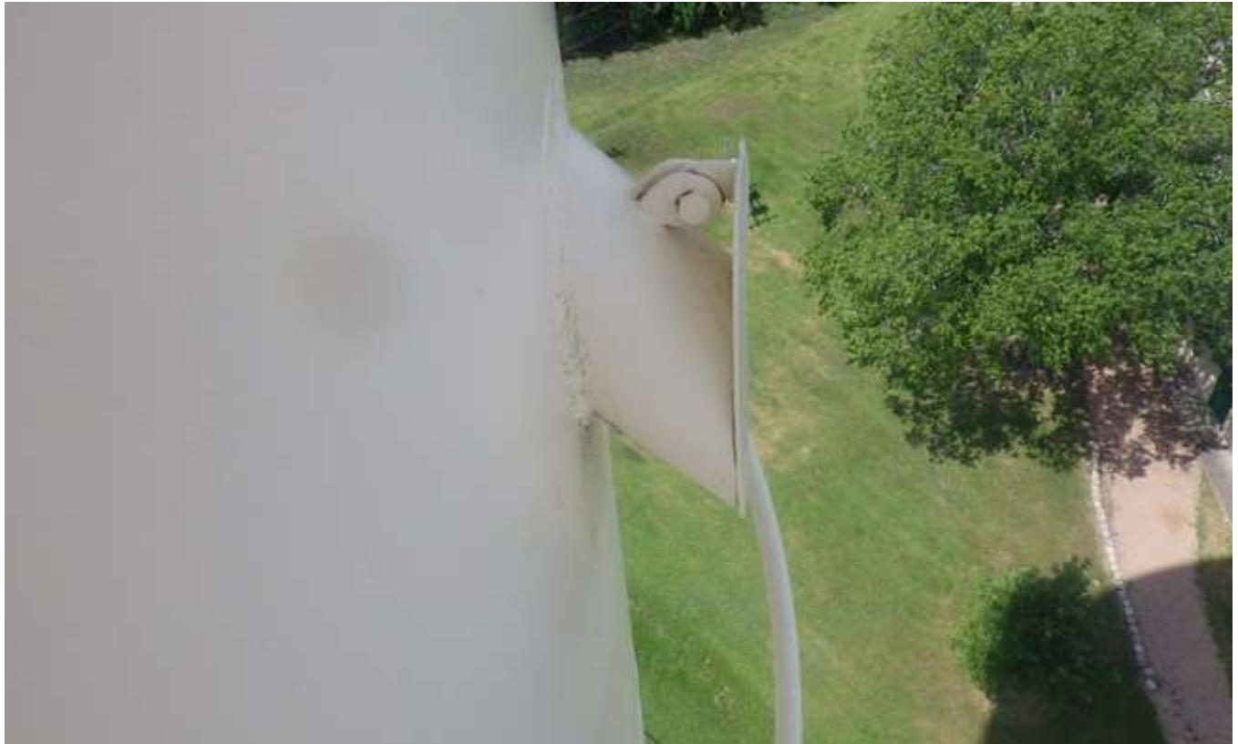
20. Stub overflow pipe discharge equipped with a flap gate near the top of the support column.
