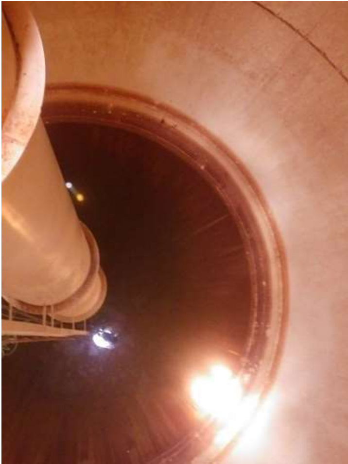
95. Interior wet access tube and bowl. Note water and silt on the bowl.
