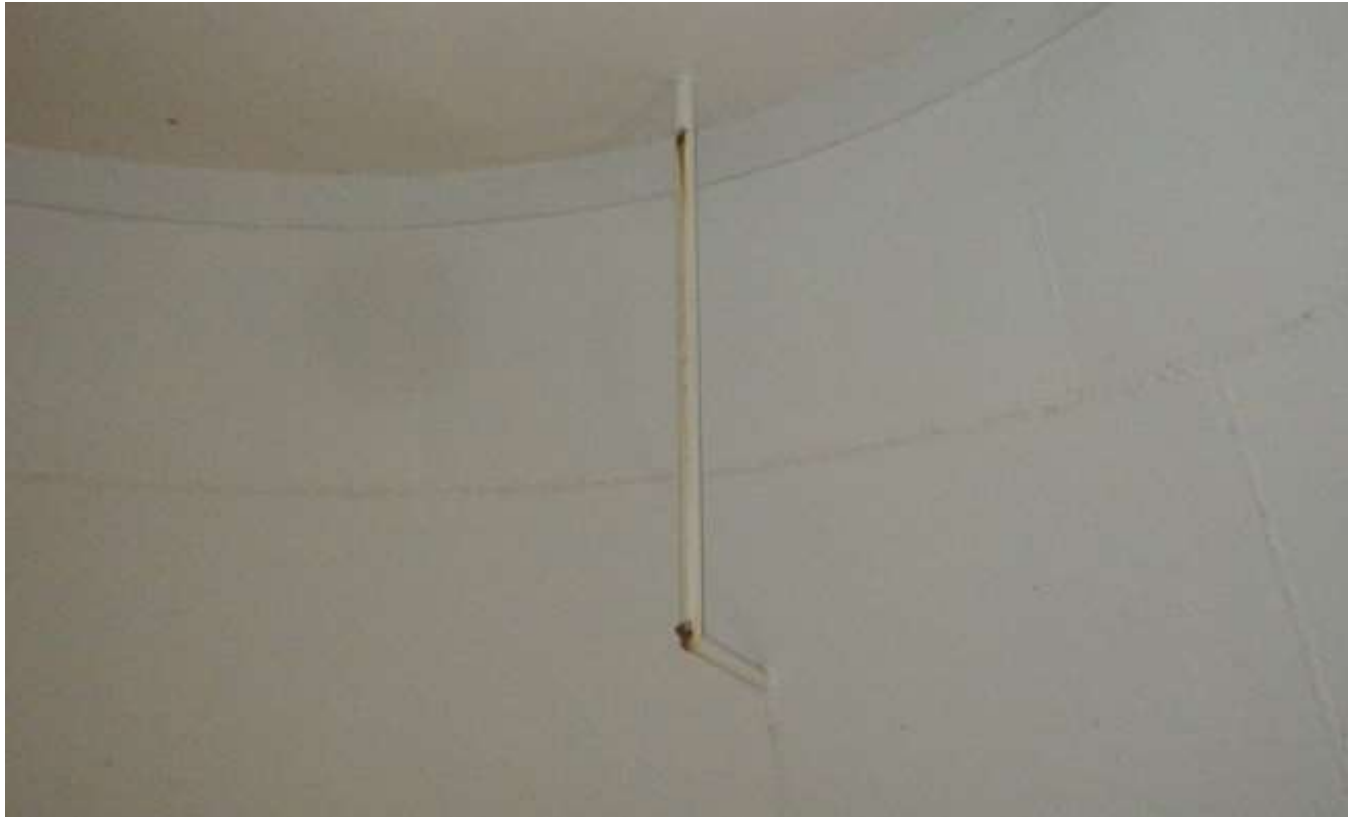
64. Spots of corrosion on the condensate ceiling drain pipe.
