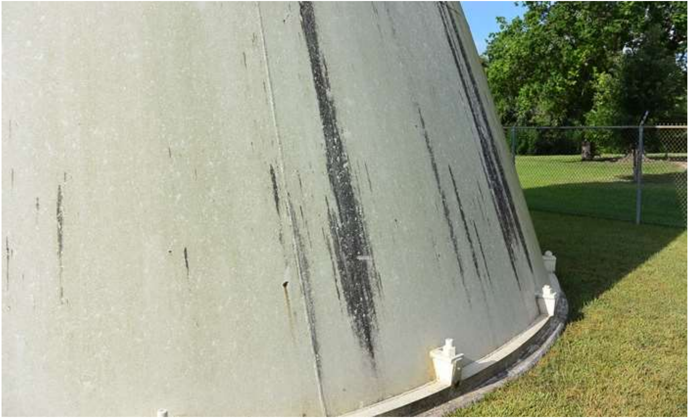
15. Mildew on the base cone exterior.
