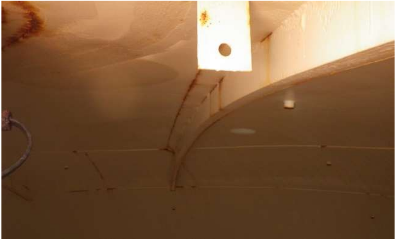
86. Corrosion and rusts staining on areas of the roof interior and stiffener. Note lug on the roof.
