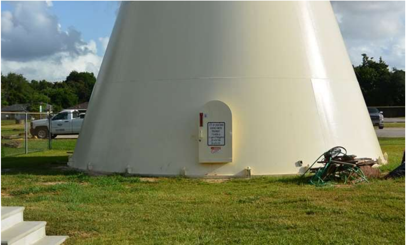
13. Base cone exterior and information and warning signs on the access door.
