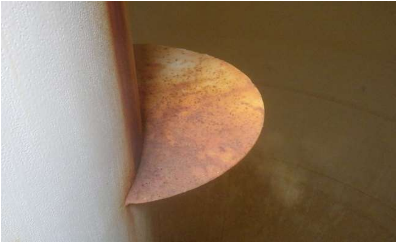
93. Corrosion on overflow inlet anti-vortex plate.
