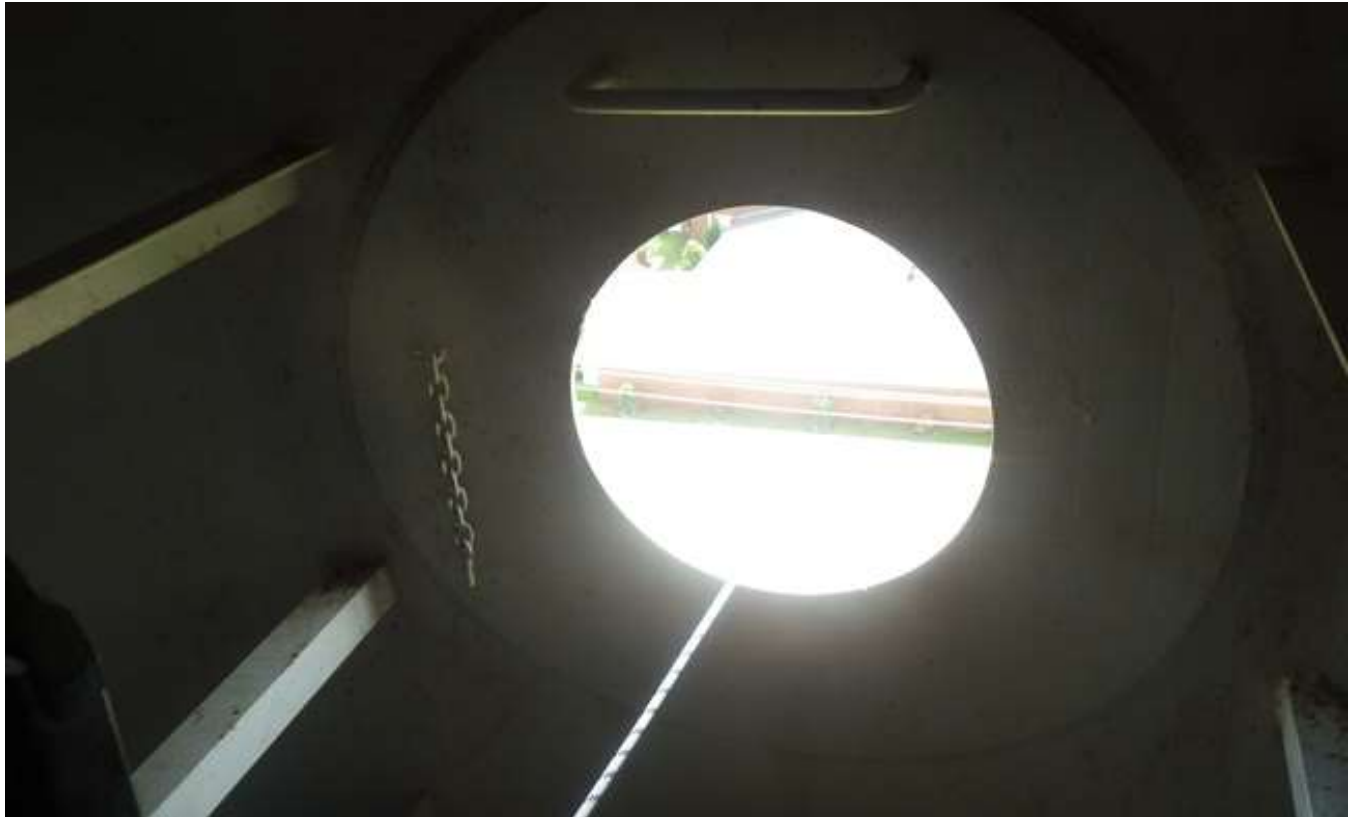
74. Painter's manhole, retaining chain, and hand hold.
