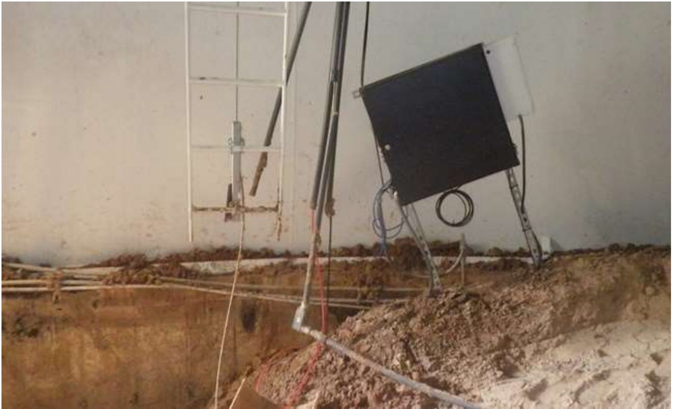
53. Electrical cabinet and broken conduits exposing wiring above severely damaged base cone floor.
