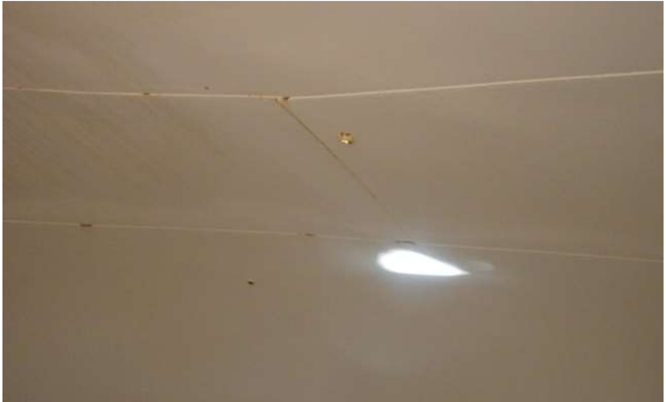
88. Minor corrosion and rust staining on areas of the roof interior.
