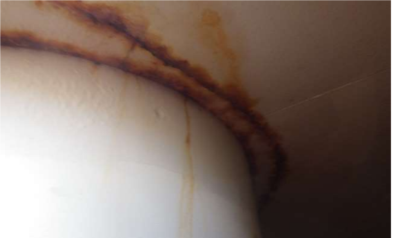
91. Corrosion and rust staining on the roof interior around the access tube.
