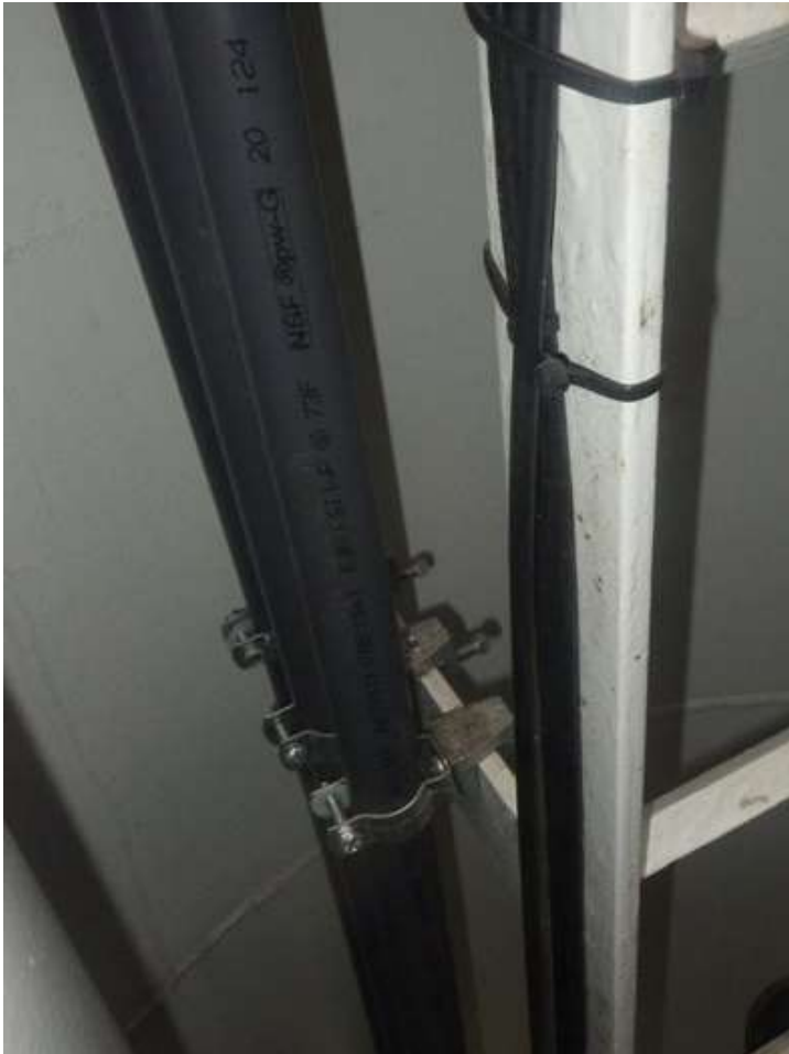
81. Cables attached to the interior dry access tube ladder brackets and side rail.
