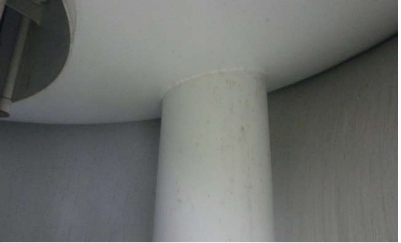
75. Inlet/outlet pipe penetrating the dry bowl.
