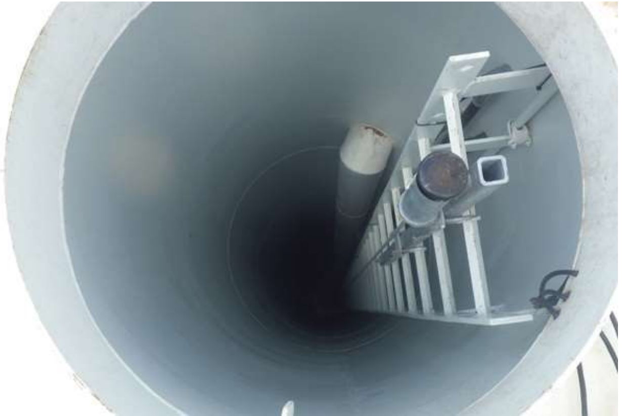
83. Overflow pipe penetrating near the top of the access tube, interior dry access tube ladder, and safe-climbing device.
