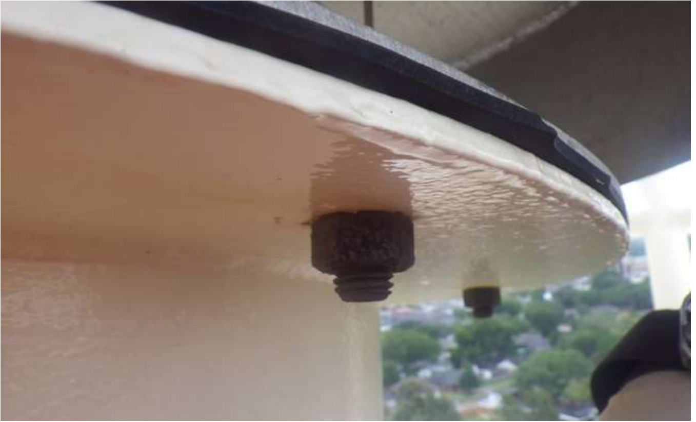
45. Gasket and corroded bolts and nuts on the roof vent flange.
