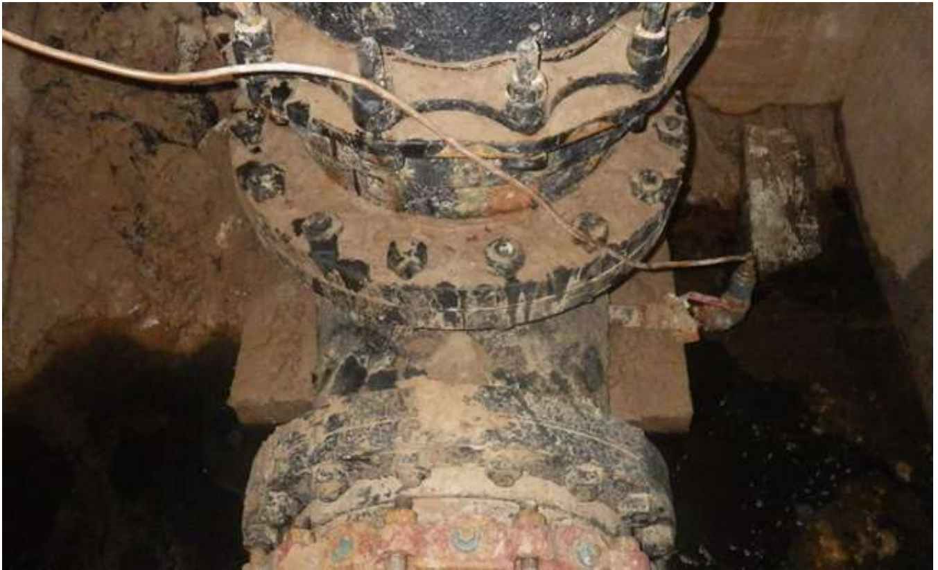
57. Piping in the pipe pit.
