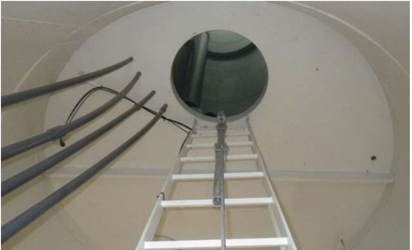
63. Base cone ladder, safe-climbing device, and cables.
