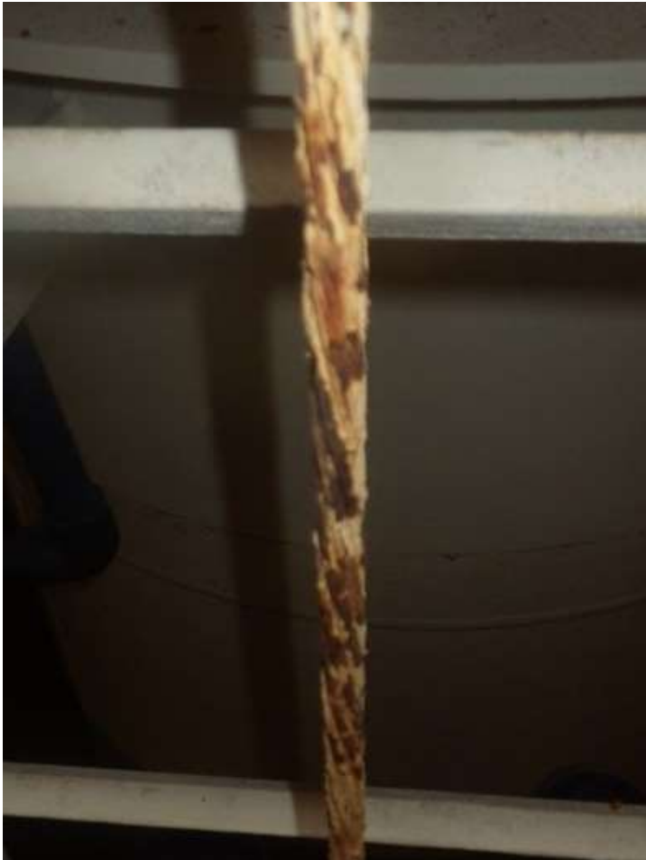
99. Corrosion on the interior wet container ladder safe-climbing device.
