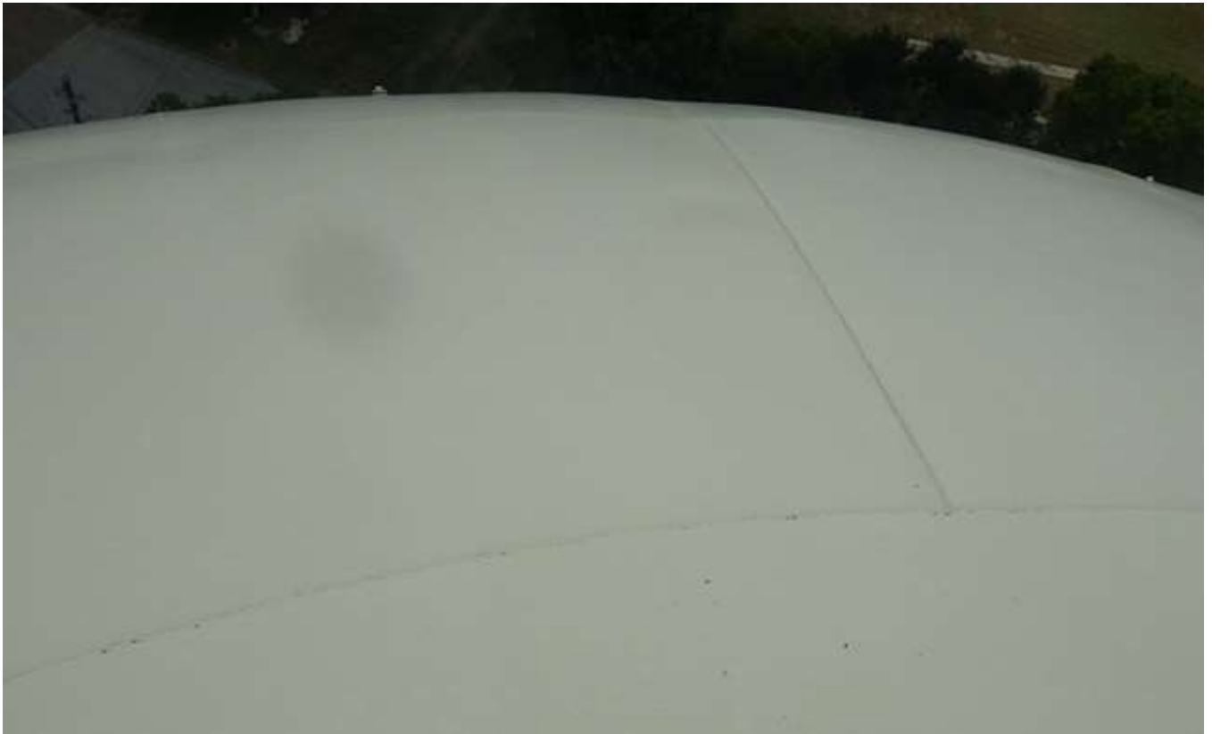
29. Irregular roof contour. Note threaded and plugged couplings in the roof.
