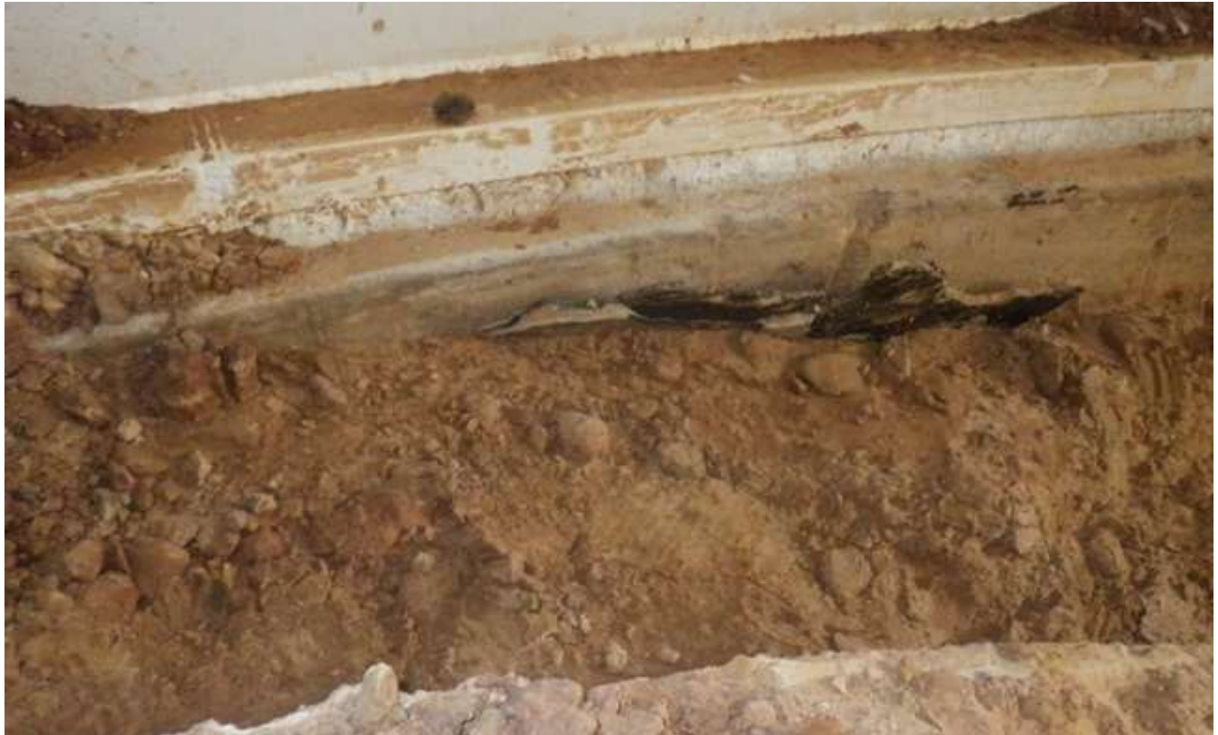
48. Severely damaged base cone floor.
