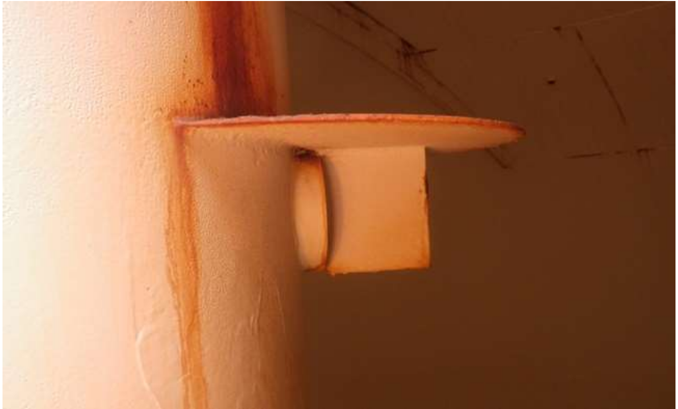
94. Corrosion on overflow inlet anti-vortex plate.
