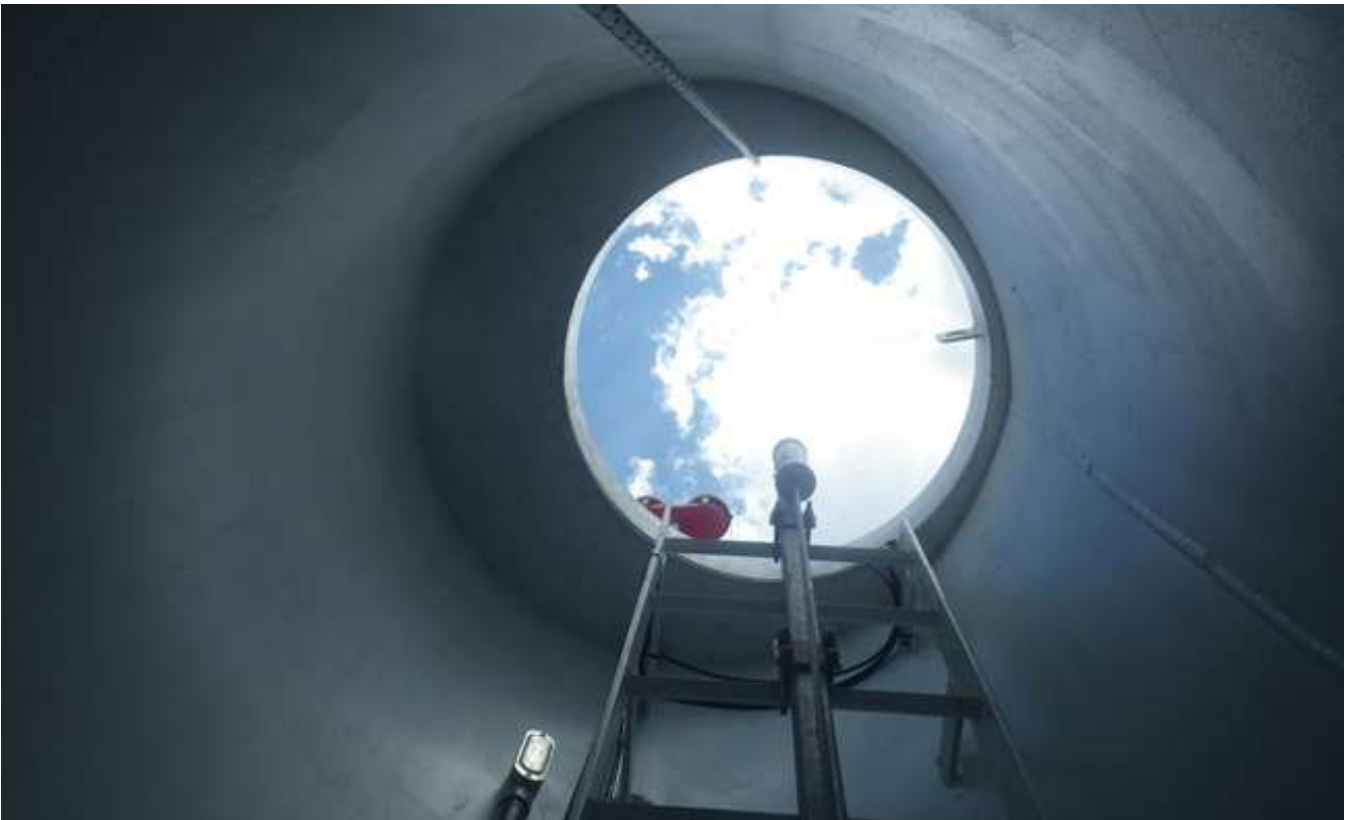
82. Interior dry access tube ladder and safe-climbing device.
