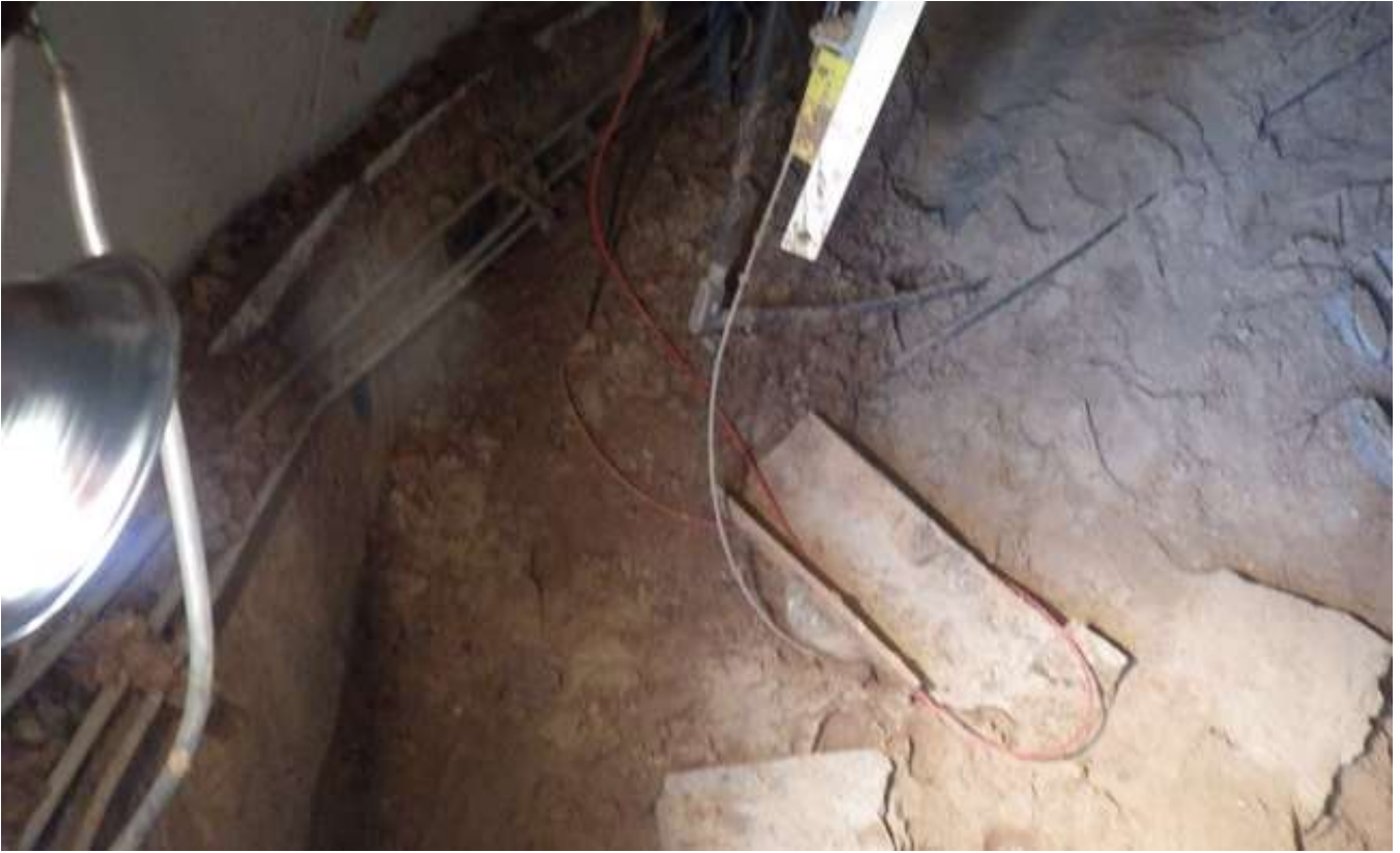
51. Debris and exposed conduits at severely damaged base cone floor.
